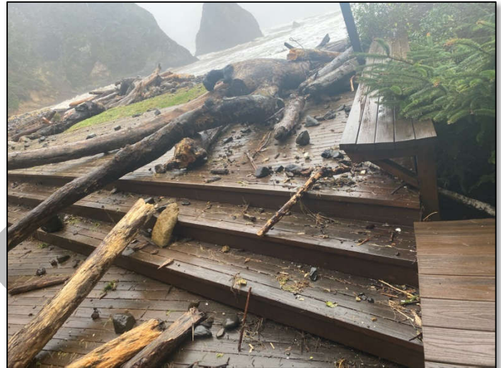
Debris Washed onto Residential Deck by 2021 Storm
